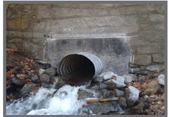
Outfall of the newly relined stone masonry culvert completed as part of the reconstruction of Route 44 in Smithfield, Rhode Island near Smith Avenue (Route 116).
